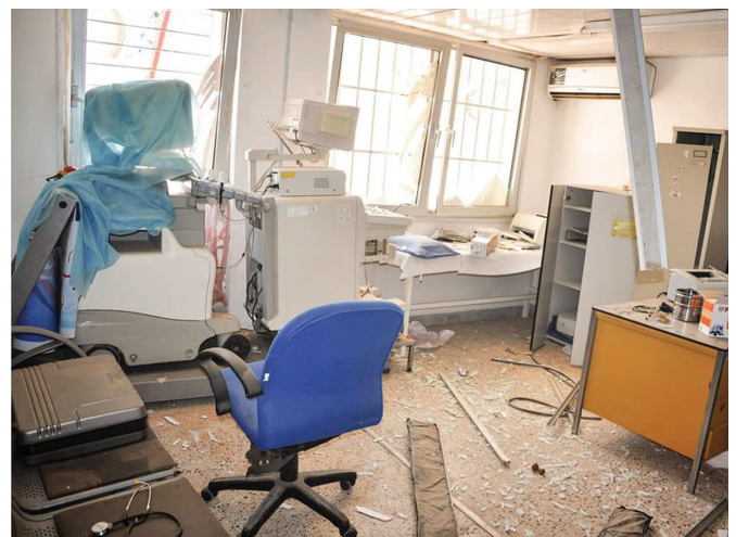
Damage to Sirt Iben Sena Hospital.
